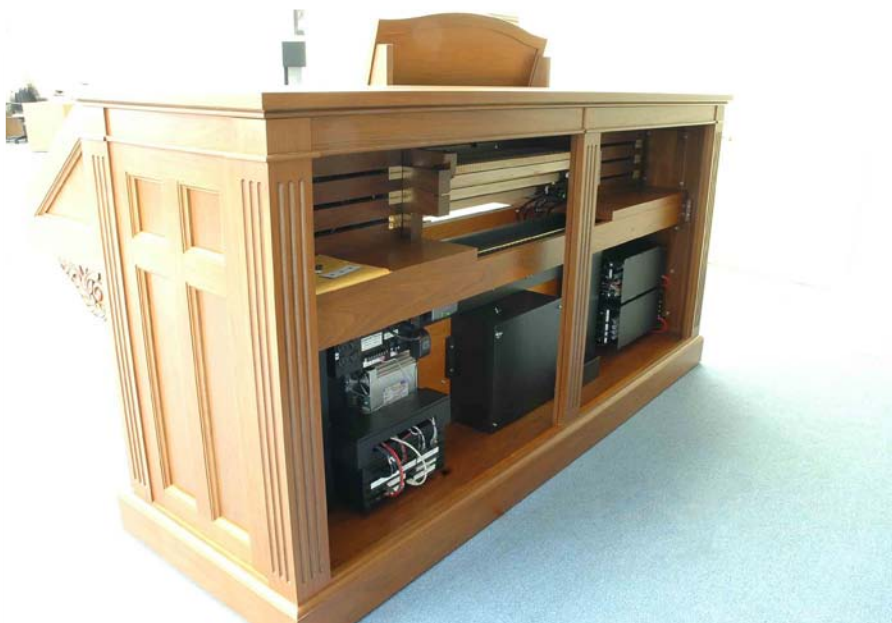
ICS-4000 Equipment Installed in a Console (photo courtesy Berghaus Organ Co)
